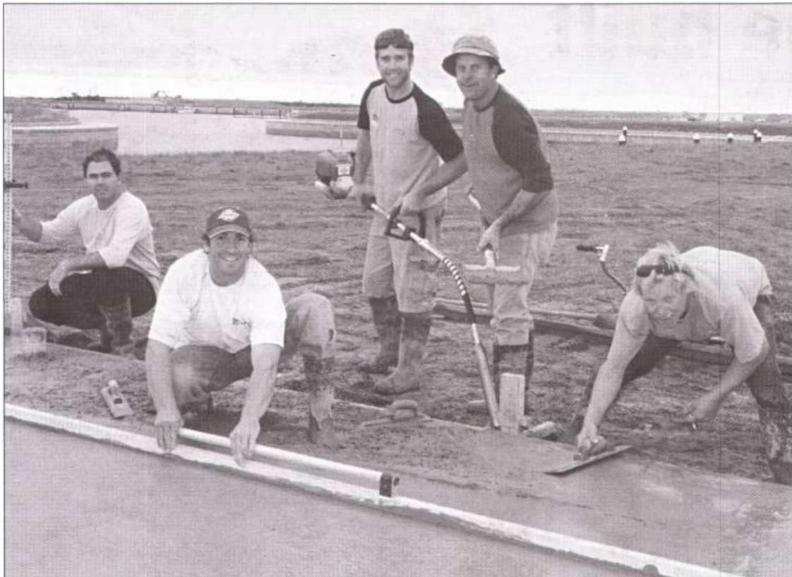
Mark Reidy (left), Casey Sharpe, Mark Gibbs, Jimmy Parker and Stevie Boyz of Hotondo Homes level the concrete on which the first home at Cape Jaffa Anchorage will be erected.
